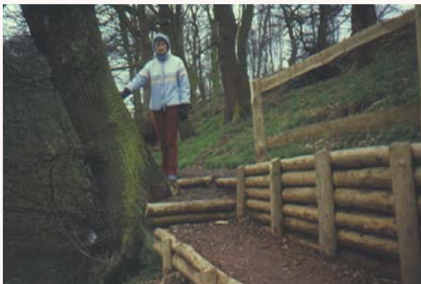
This photograph shows erosion control and access work. A revetment helps to stabilise the bank and steps prevent it from being eroded as people climb it
